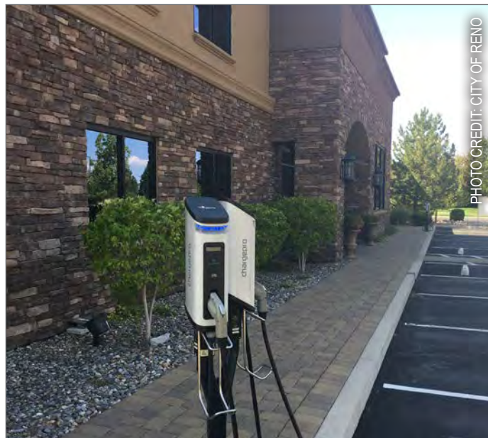
Example: Electric vehicle charging stations
